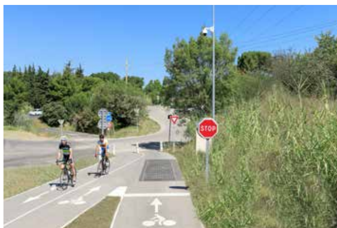
A 12-panels Wattway Pack provides autonomy to a high-definition surveillance camera and its communication router
